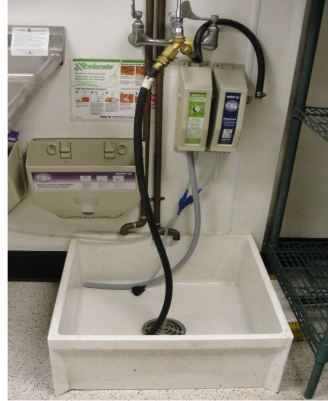
Curbed Cleaning Facility
