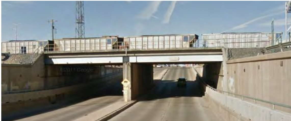
A look at the SE 10 th overpass, deemed a high priority historic resource. Source: Google maps, ©2013, maps.google.com
