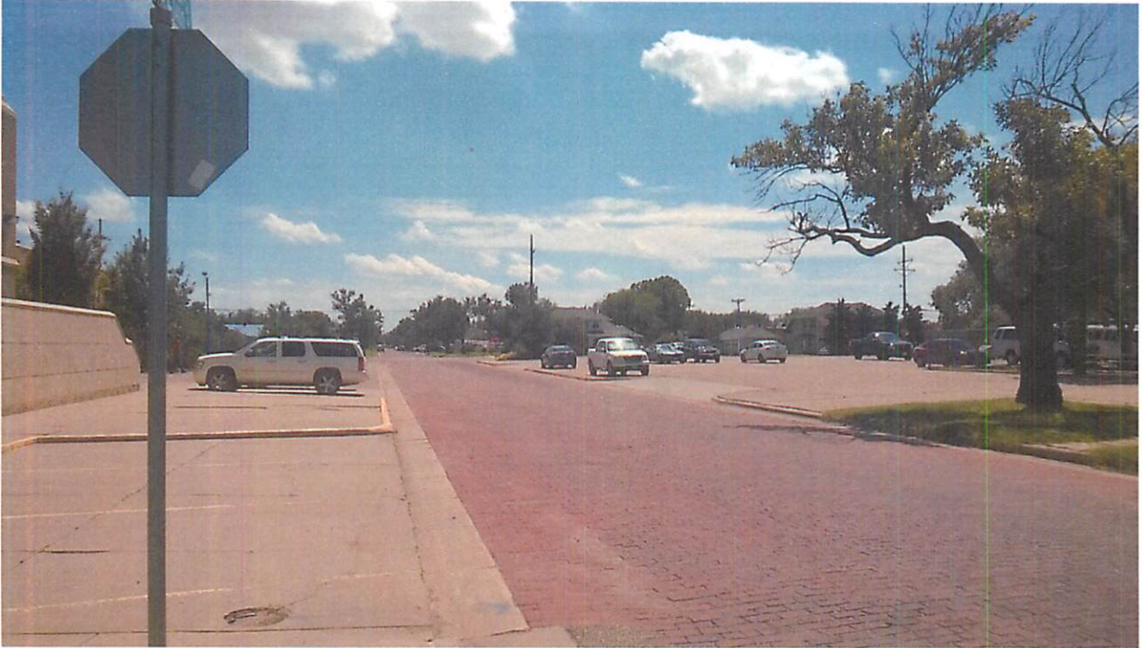
Looking southwest down S Monroe St, which is 80' wide of ROW. Bricks are to be recycled.
