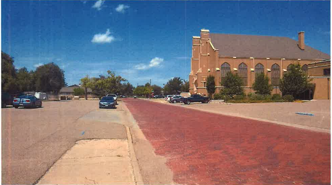
Looking northeast up S Monroe St, which is 80' wide of ROW. Bricks are to be recycled.
