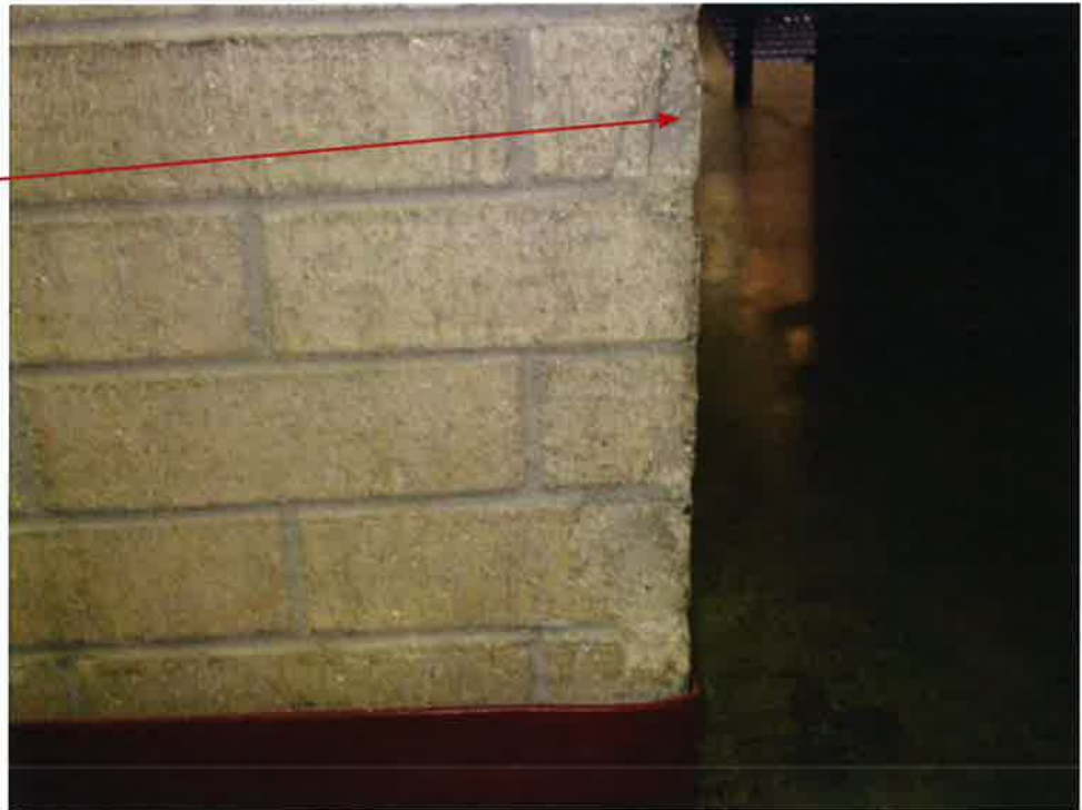
Damage to brick at Coliseum vomitory
